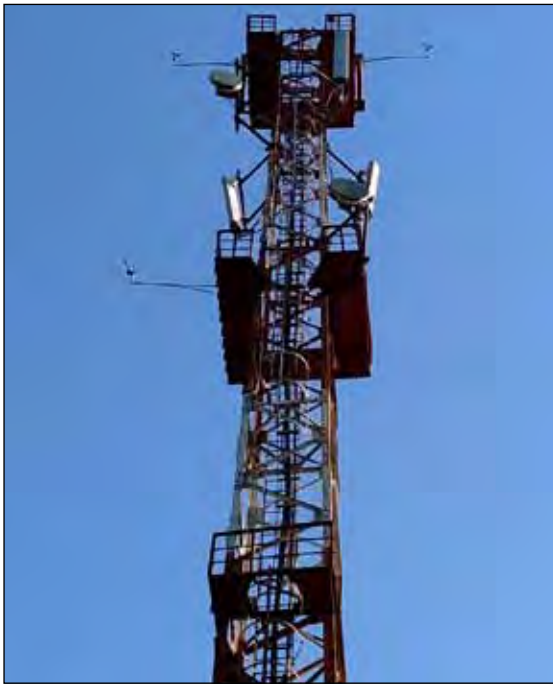
Figure 5: Wind Measurements Using Telecom Towers
