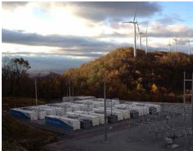
Figure 2: AES Laurel Mountain facility with 32 MW Li-Ion batteries @ 110 MW wind farm (Source: AES)
