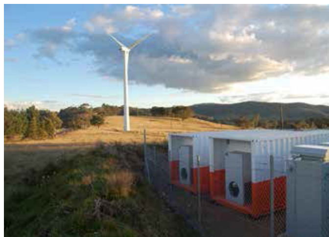
Figure 5: Ecoalt Battery at Hampton Wind Farm in NSW
